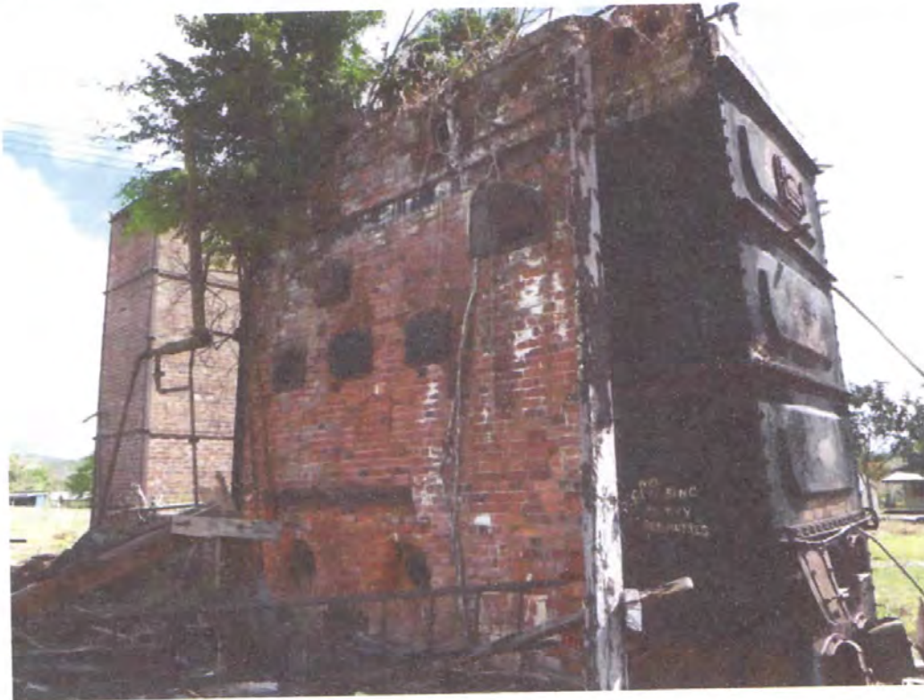
Figure 19 Left side of the Stirling boiler. Visible are the access doors to allow the tubes to be cleaned of soot, and to allow inspection of the boiler. Obscured by the tree growing at the back of the boiler is the additional steam drum, and the main steam pipe is also visible to the left. In the foreground is the access ladder which original stood by the boiler allowing access to a platform (no longer present) (September 2010)
