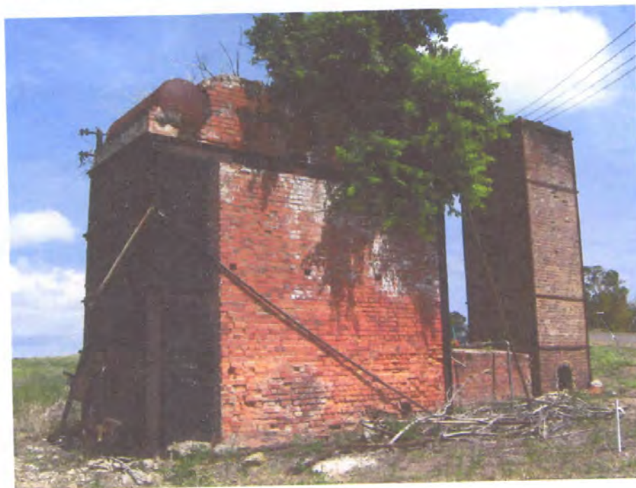
Figure 25 Right hand side of Stirling water tube boiler. The boiler furnace doors are to the left. To the right the flue exits the base of the boiler and passes to the base of the chimney. Two of the steam drums are visible at the top of the boiler. (September 2010)
