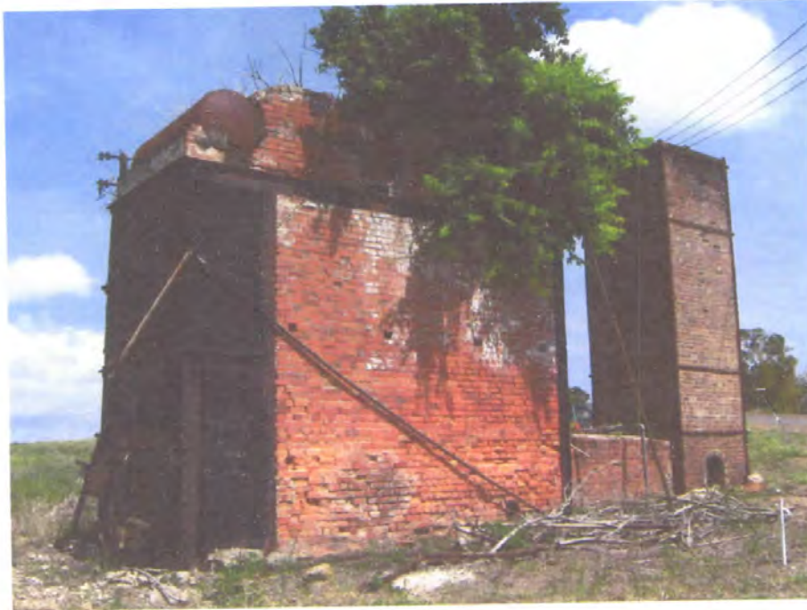
Figure 25 Right hand side of Stirling water tube boiler. The boiler furnace doors are to the left. To the right the flue exits the base of the boiler and passes to the base of the chimney. Two of the steam drums are visible at the top of the boiler. (September 2010)
